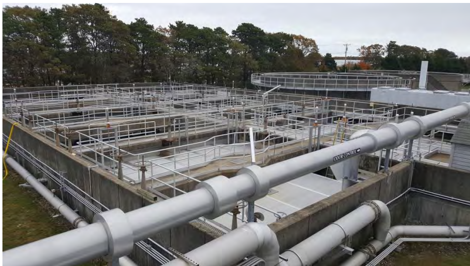
Middle and South Aeration Tanks
