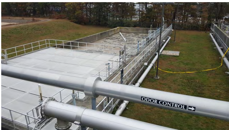
North Aeration Tank
