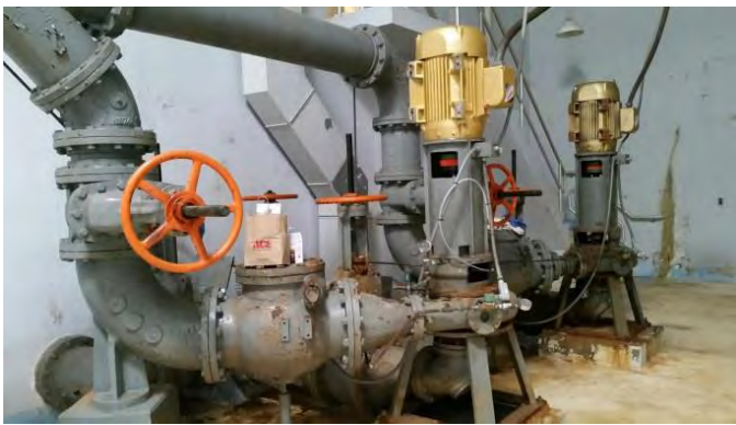
Freezer Road Pump Room
