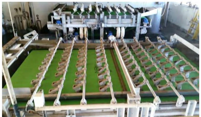
Sludge Thickening Belt
