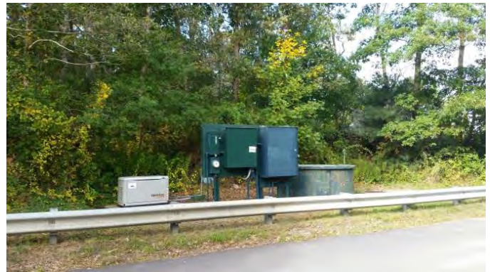
Oak Neck Road Pump Station
