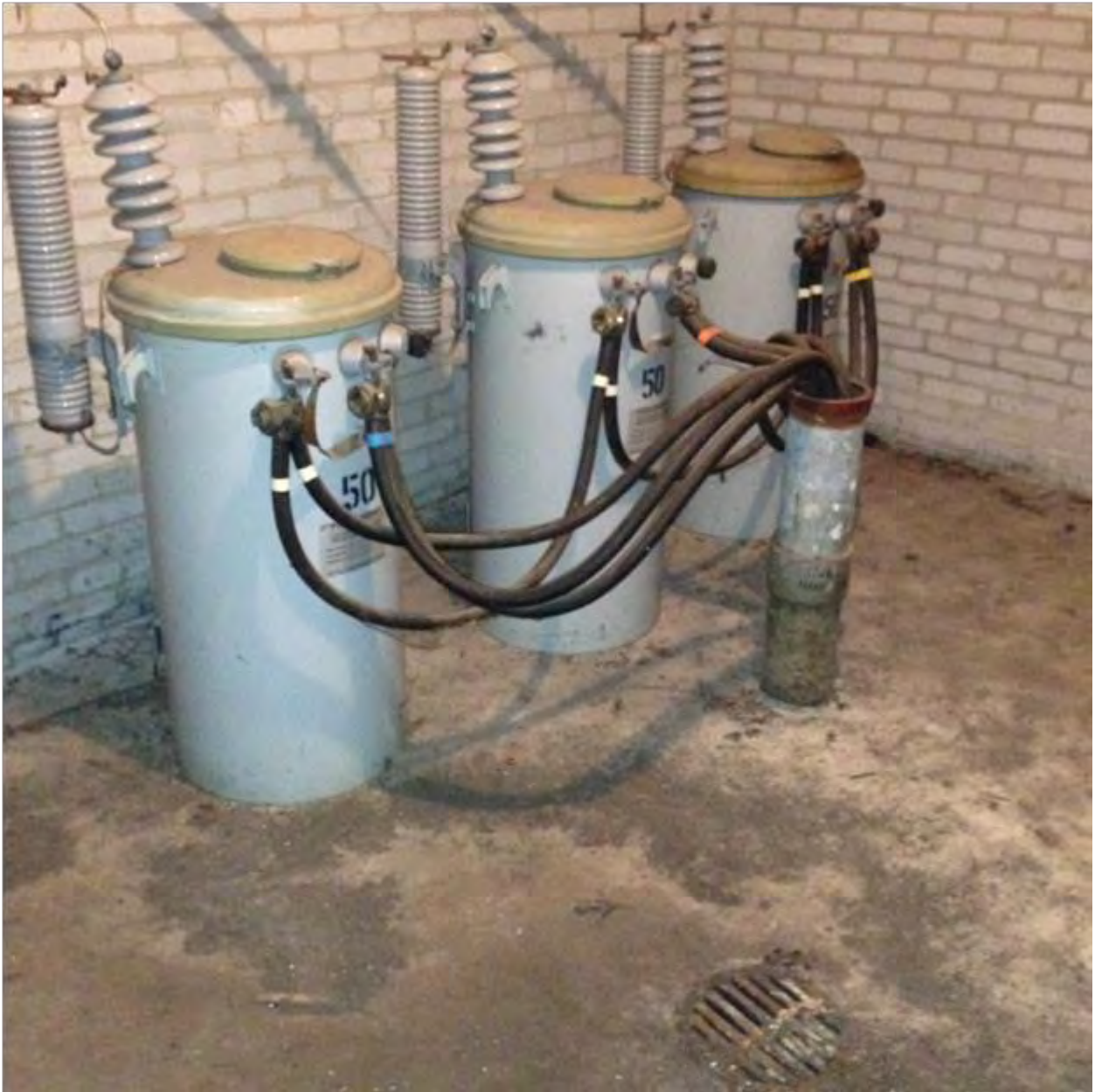
Typical Underground Transformer Vault
