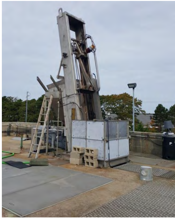
Mechanical Bar Screen
