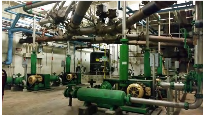
Septage Blower Room
