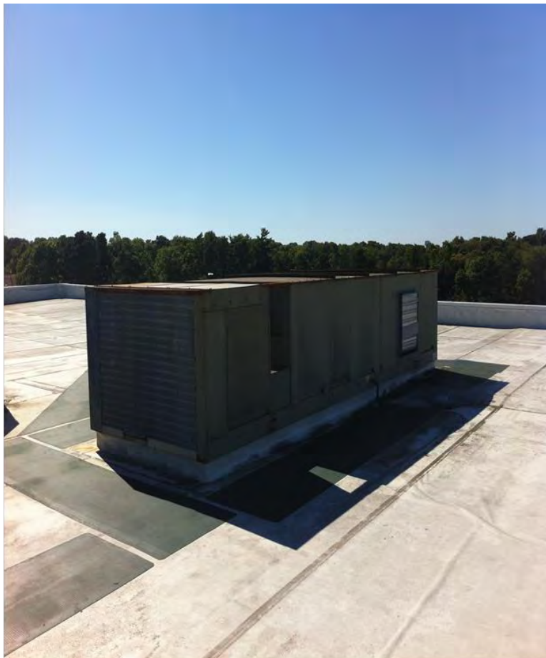
Roof Top Units (RTU)
