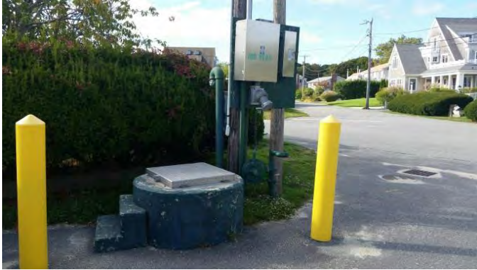
Bayshore Road Pump Station
