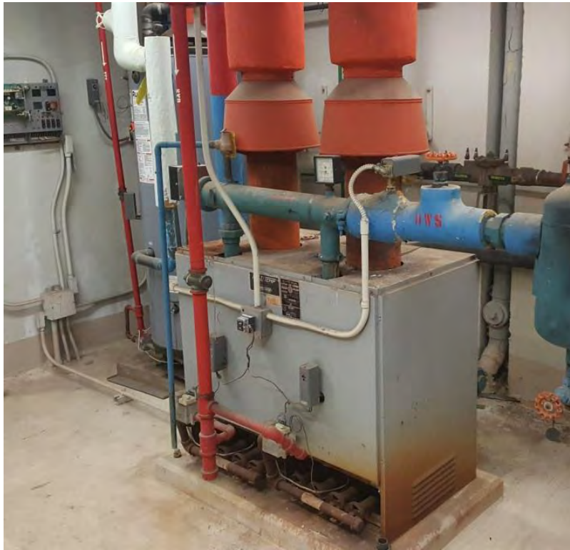
Mechanics Building Boiler
