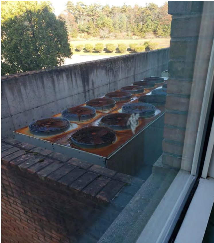
Barnstable United Elementary School Chillers
