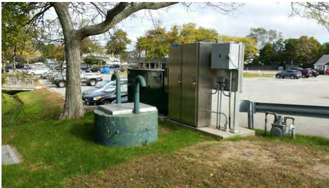
720 Main Street Pump Station
