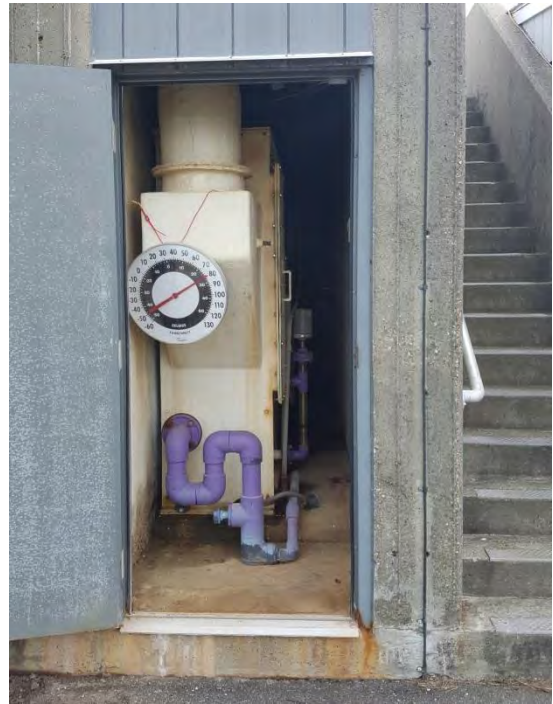
Odor Control System Access
