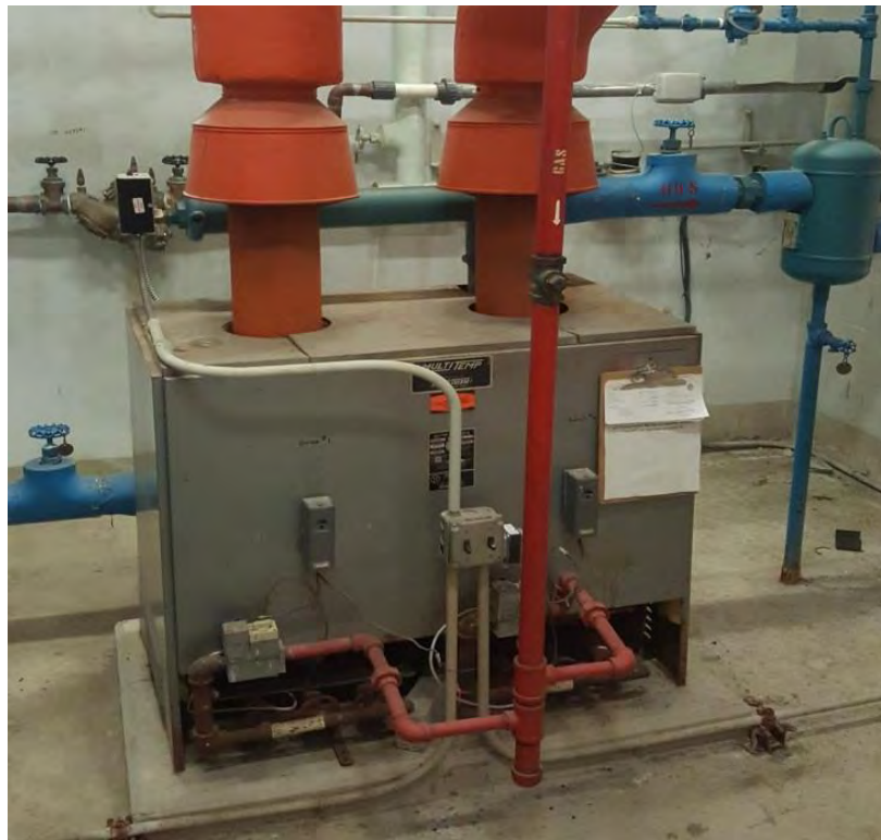
Control Building Boiler
