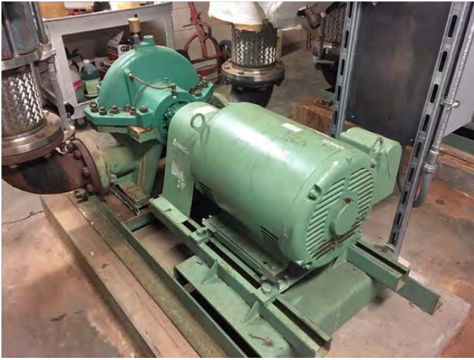
Typical BHS Pumpset
