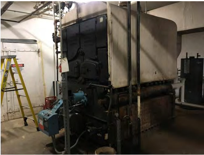
Barnstable West Barnstable Elementary School Boiler
