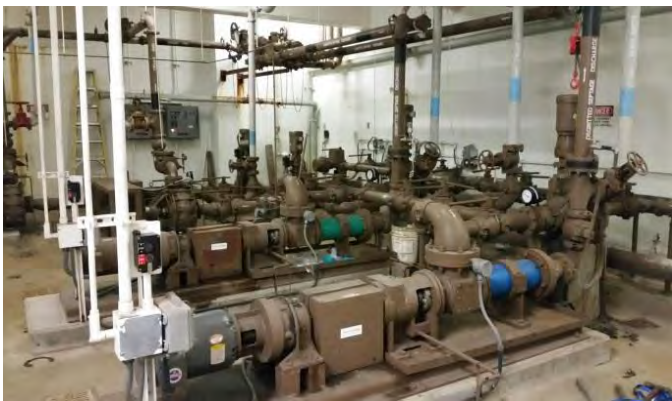
Sludge Pump Room
